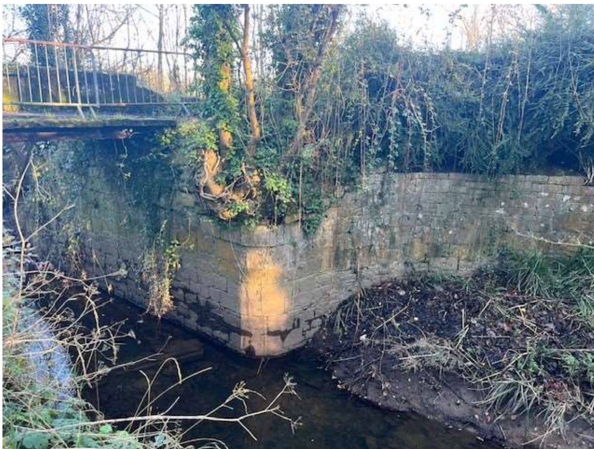
Plate 12-19: Bridge 3 showing vegetation around abutment walls and collapsed parapet
