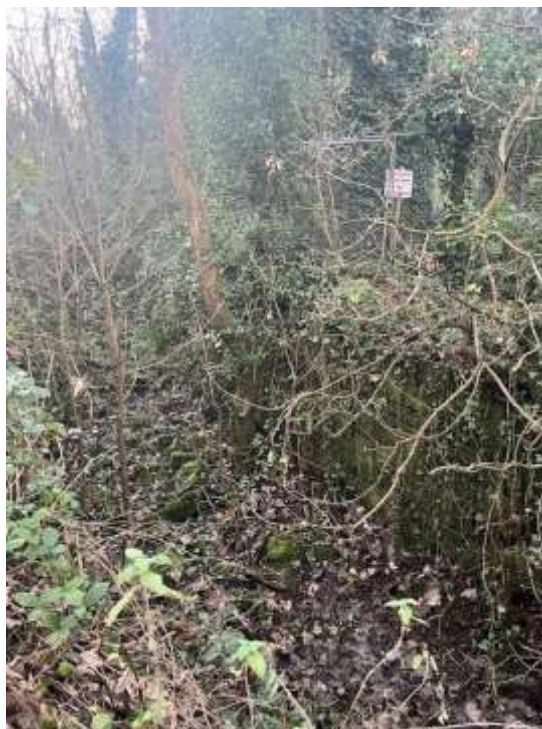
Plate 12-7: Mill Race immediately east of Plassey Mill tower. Masonry walls either side very overgrown
