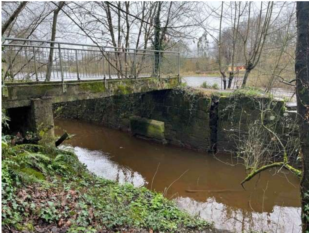
Plate 12-20: View of Bridge 5 from the east showing deck resting on historic masonry
