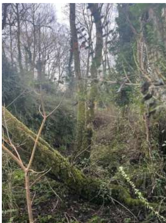
Plate 12-8: Mill Race immediately east of Plassey Mill tower. Masonry walls either side very overgrown.
