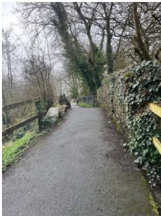
Plate 12-17: Bridge 2 looking East, parapet wall to the south with missing masonry & capstones
